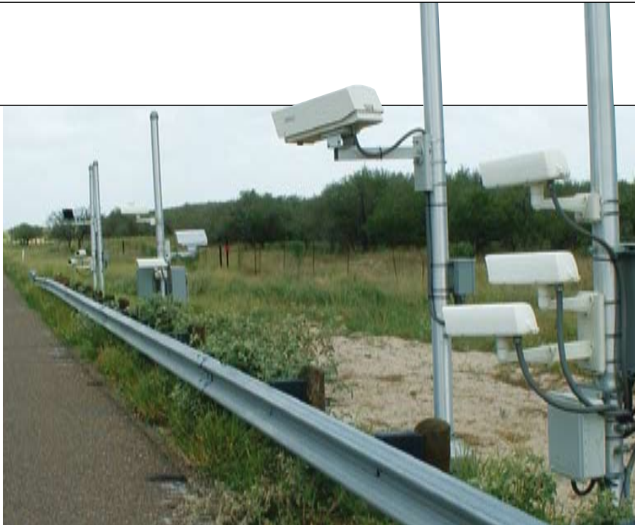
📌 Image data can be captured and then archived for later analysis in order to spot traffic trends
